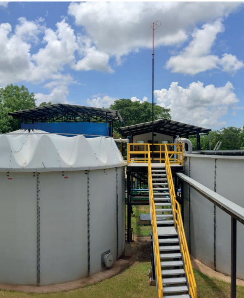
Wastewater treatment plant of the Cold Cuts Business in Aguachica, Colombia.
